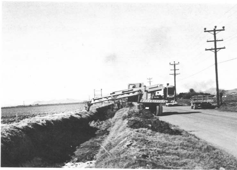
Figure 16. Aquatic weeds and silt being removed from an unlined lateral by an all-hydraulic type. Photo PX-D-60891.
