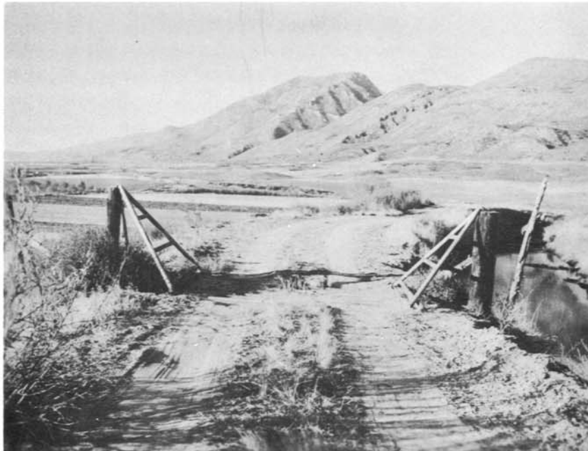
Photo 9 - Typical pit type cattle guard used on the operating road of the Provo Reservoir Canal, Provo River Project, Utah
