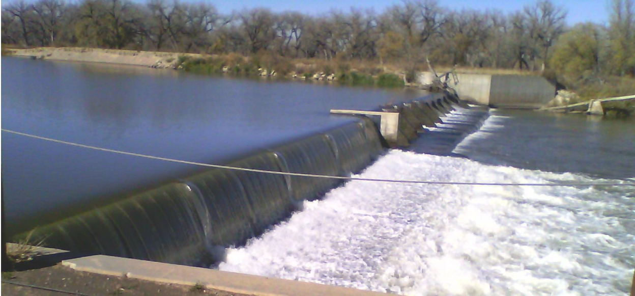
Figure 5 Photo of a Similar Pneumatic Gate Diversion Dam
