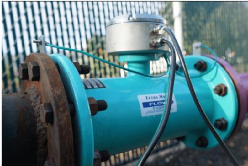
Figure 5 – Installed Magnetic Smart Meter
