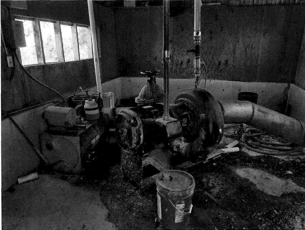
Figure 6: King Pump Station
