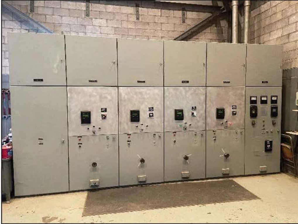
Figure 3 Existing pump station drives do not allow variable speed operation
