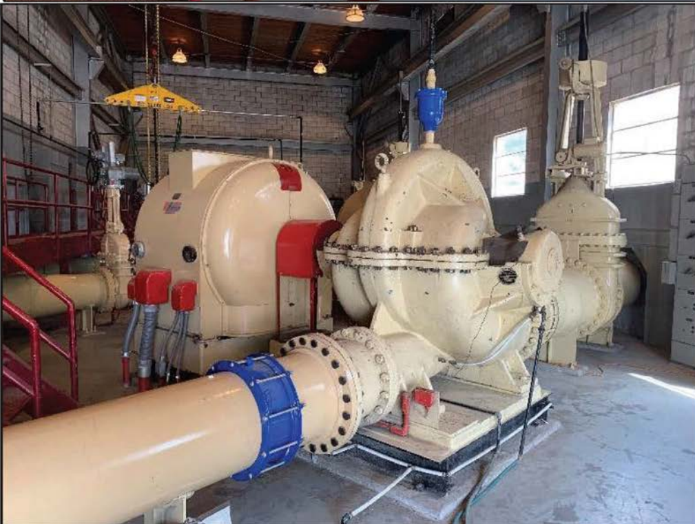
Figure 2 Existing 3700 Hp pump station (top) and 1250 Hp pump (bottom)
