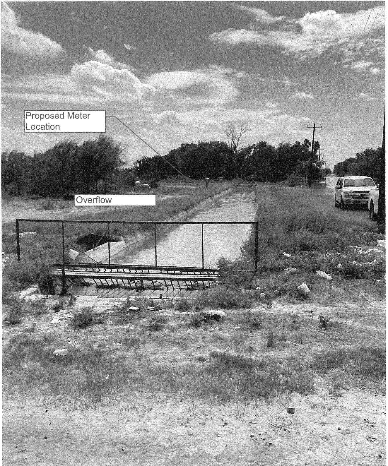
Figure 4 Engelman Irrigation Solar Powered Metering and Overflow Monitoring Location
