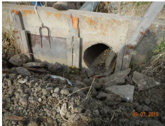
Old headgate with old slide unit AND without any gate
