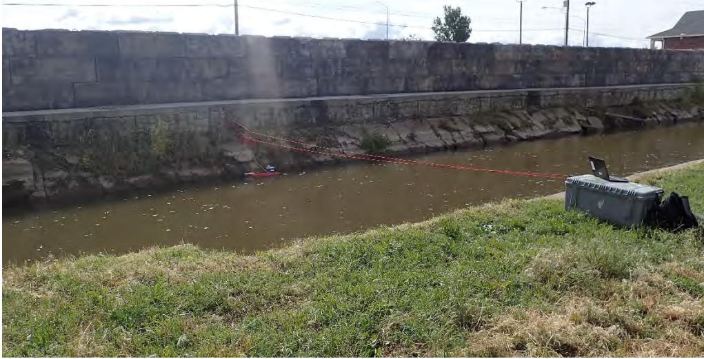
Figure 7 - Upstream measurement location. Note vegetation growing in cracks of fractured concrete liner. ADCP is in boom position.
