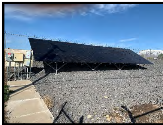
Photo 5 Existing Solar Array
