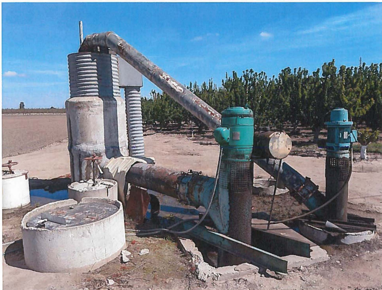
Figure 4. Area 18 Pipeline Existing Pump System, View from the South. The green pump is 20 hp while the blue pump is 10 hp.
