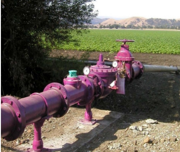
Figure 5 Recycled Water Turnout in South Santa Clara
