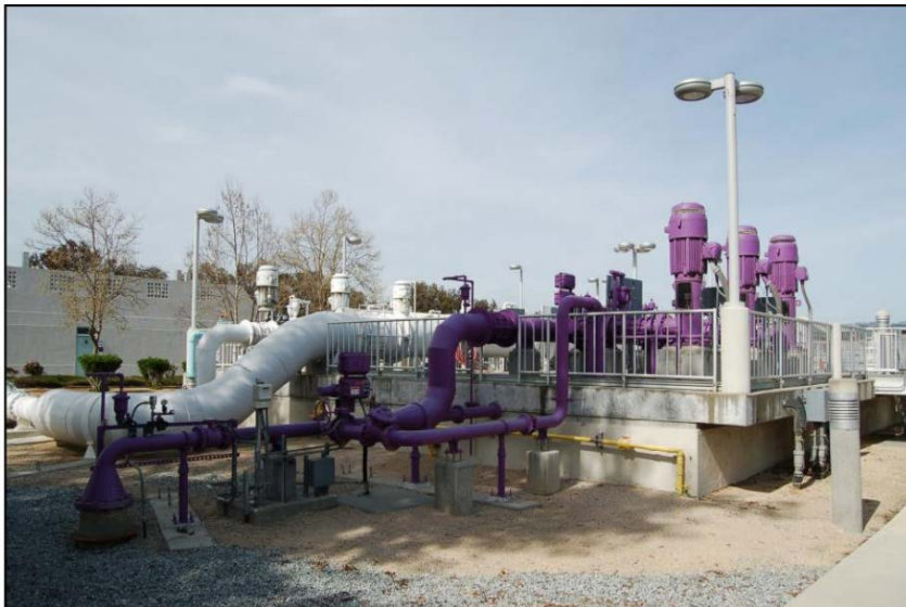
Figure 2 SCRWA WWTP & Recycled Water Pumps
