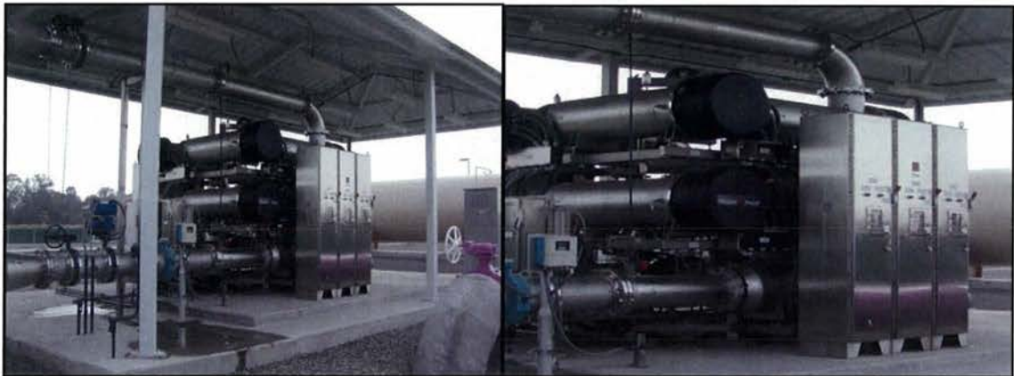
Existing UV System
