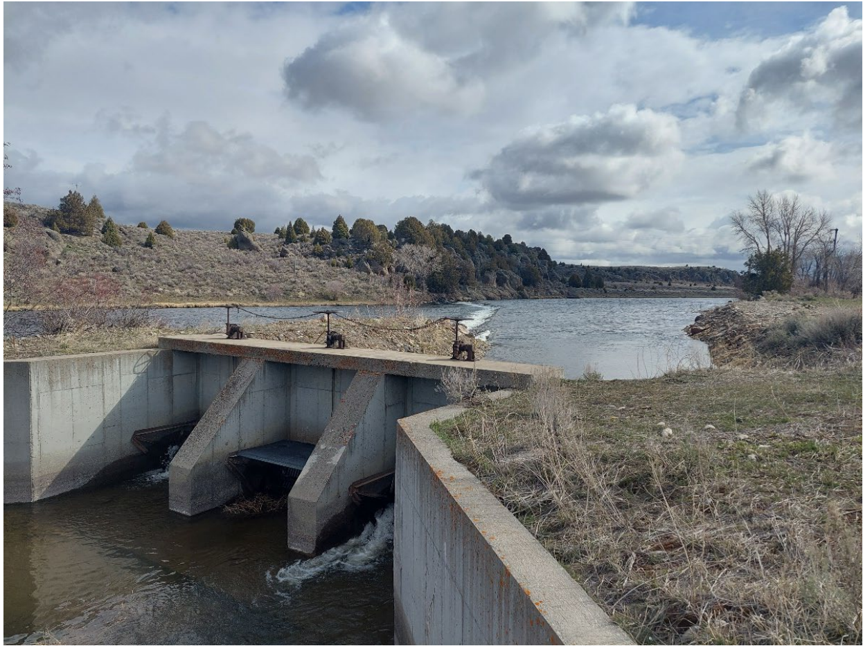
Enterprise Irrigation District Canal Headgate
