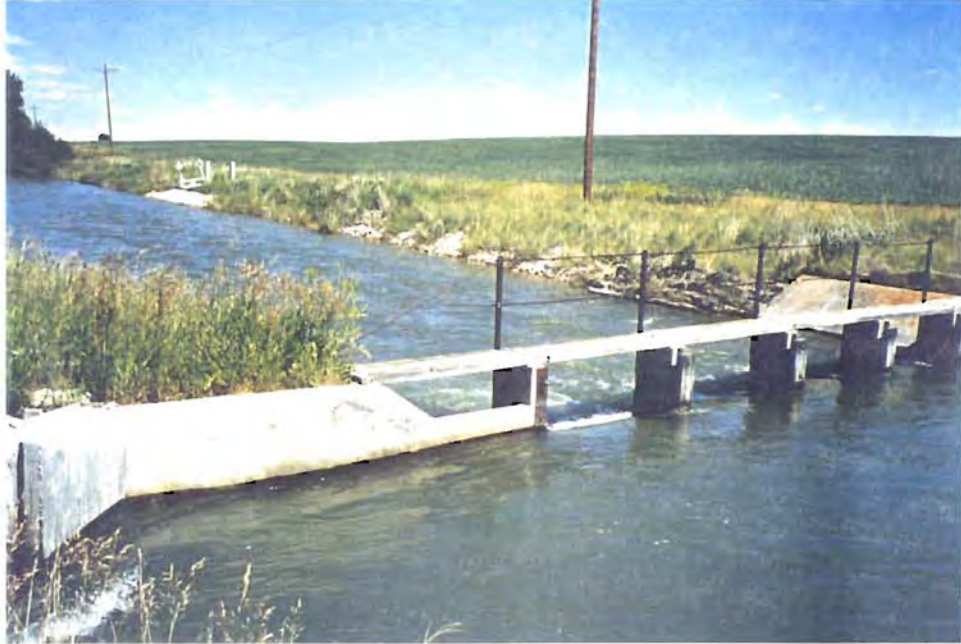
Photo 11 - GSC Check 2 (Johnson Drop), MCC headworks
