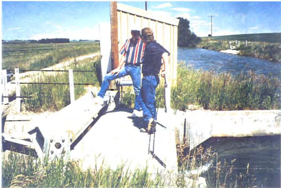
Photo 12 - Radial gate at inlet to Johnson Drop (GSC Check 2)
