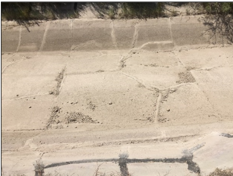
Photo 3: Existing conditions of main canal within the project area, near Jayders Rd. Note: cracks webbing across the canal and the accumulated rubble and sediment where the concrete has settled.
