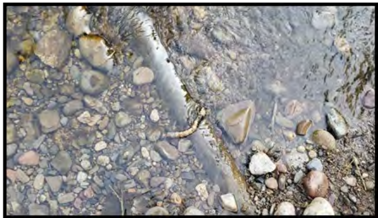
Figure 5. Exposed utility pipes running across the streambed of Warm Springs Creek.
