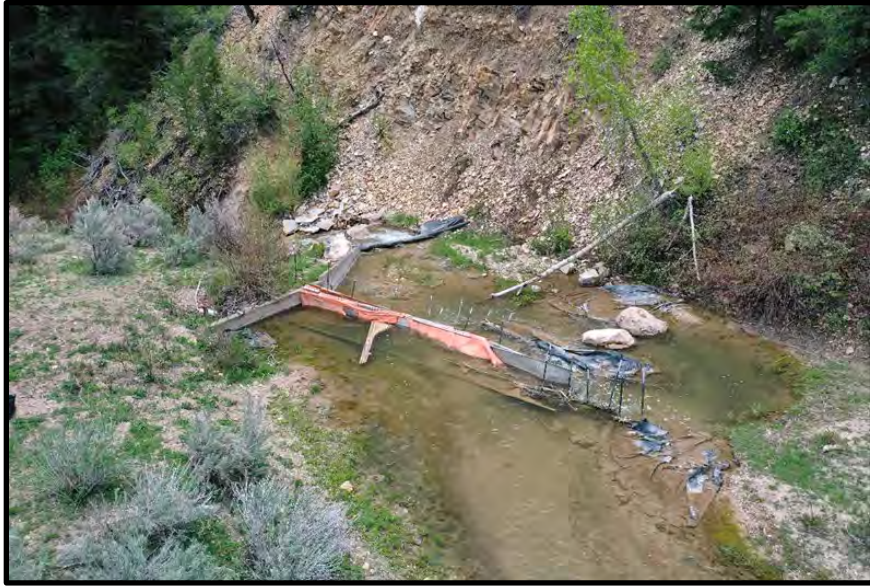
Figure 5. A new fish barrier will support native fish habitat, eliminate non-native fish species, and eliminate the annual construction of a pushup dam.
