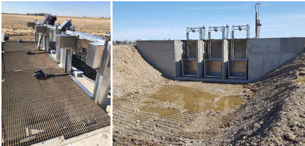
Phase 1 – Smart Check on GM-100 Constructed by GID (2020-2021) and Partially Funded by WaterSmart Grant
