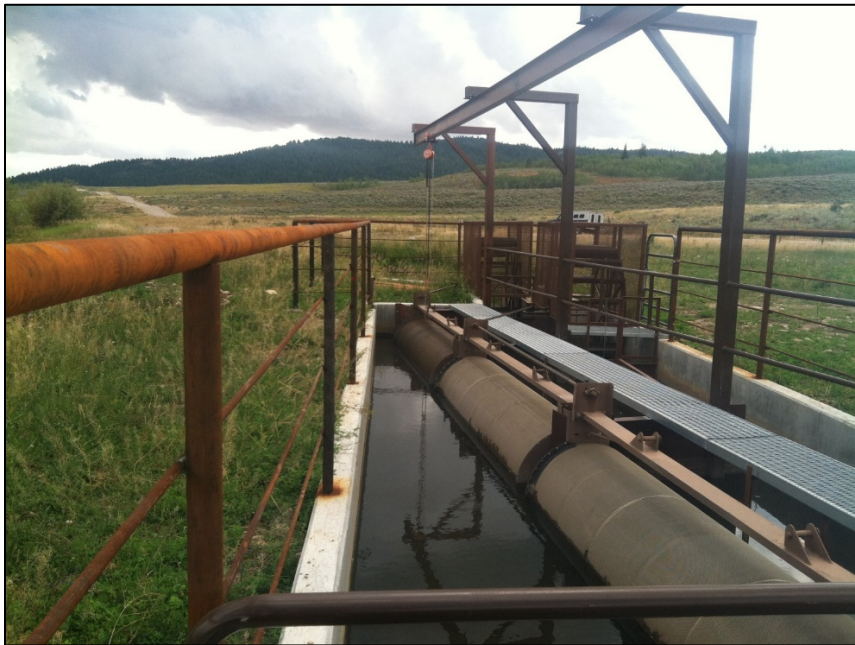
Figure 6. Photo of the Treasureton Diversion fish screen installed by Trout Unlimited on Cottonwood Creek (Idaho) in 2014. Three rotary drums (12' length x 36" diameter) are turned by two paddlewheels (the lower wheel drives the lowest-drum, and the upper wheel drives the top two drums). The screen was designed for a maximum diversion rate of 40 cfs. A similar type and size of screen is being considered for the new irrigation diversion on Paris Creek.
