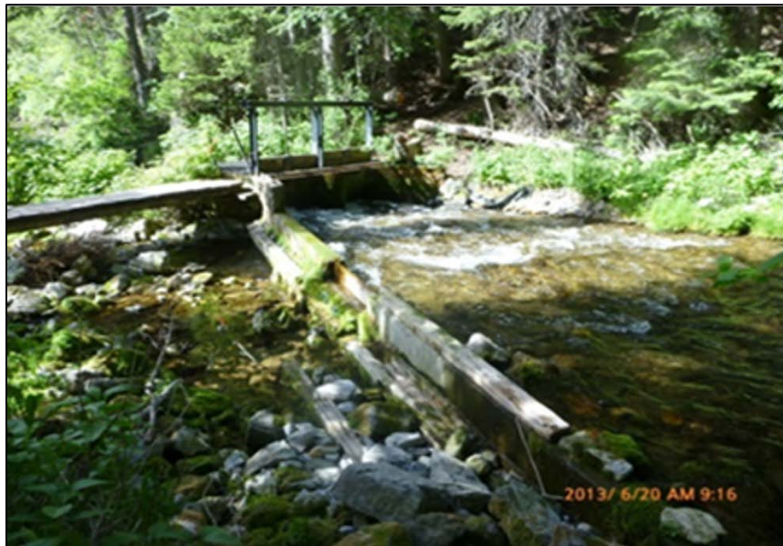
Figure 2. Photo of the diversion structure for the power canal during June 20, 2013. The log timbers and headgate will be removed as part of the decommissioning process. Note that most of the streamflow is being directed into the headgate and power canal with little stream flow downstream of the diversion structure.
