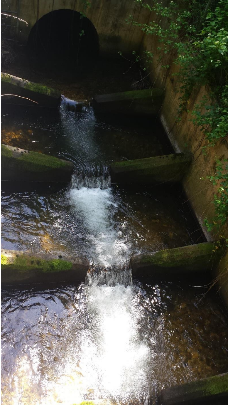
Pool and chute fishway Cement Ck near Naselle.
