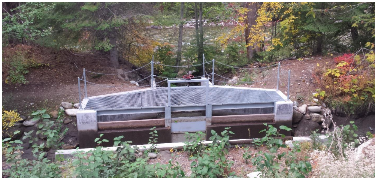
Looking at the spill portion of the structure out towards the river. The checkboards are pulled at the end of the season to help flush/draw sediment out of the ditch and run it back to the river.
