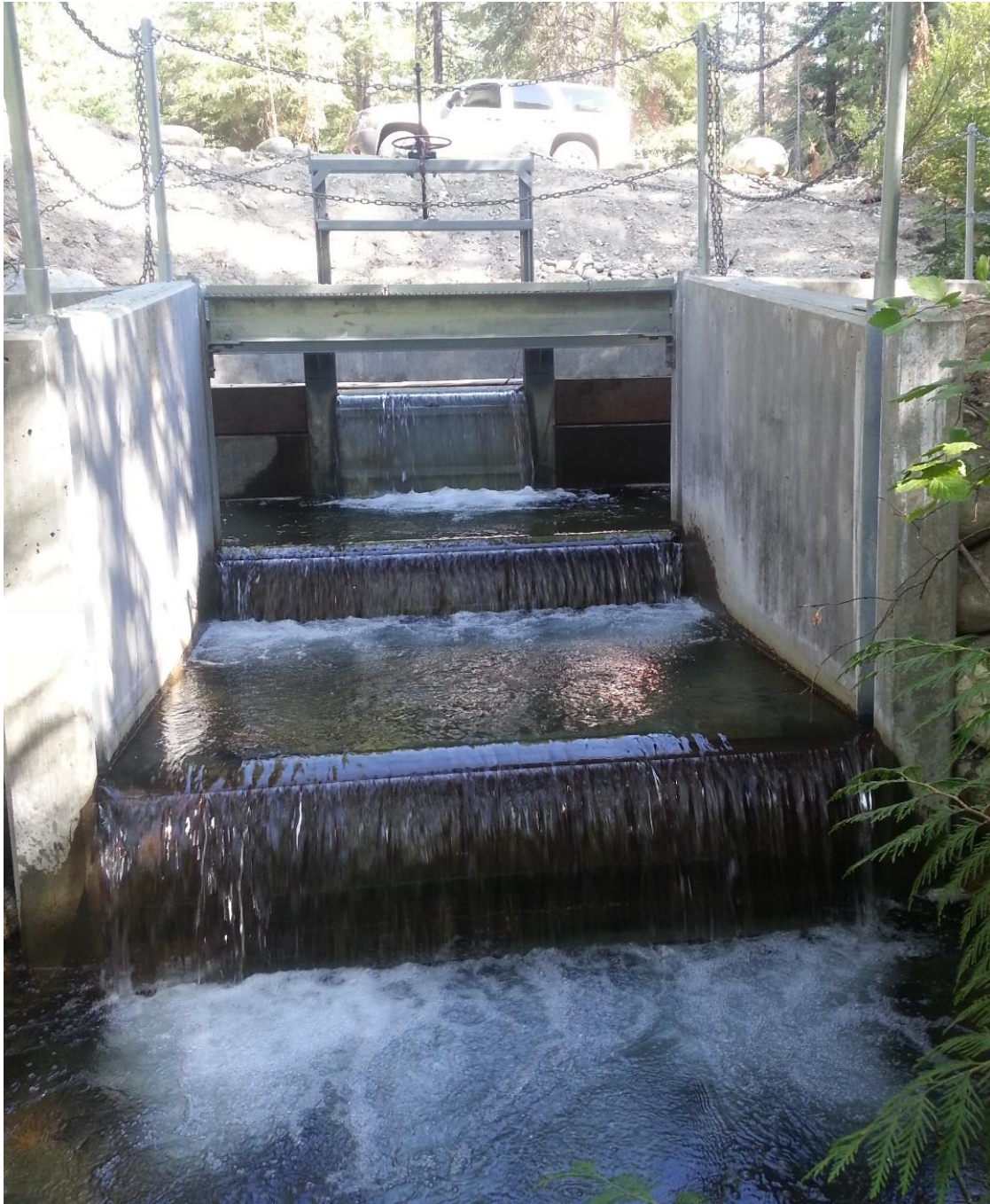
A view from the downstream end of the spill structure up towards the ditch.
