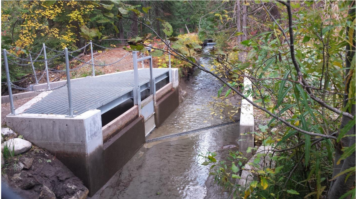
This is an example of a spill structure looking upstream along the ditch alignment off the Chiwawa River near Plain.
