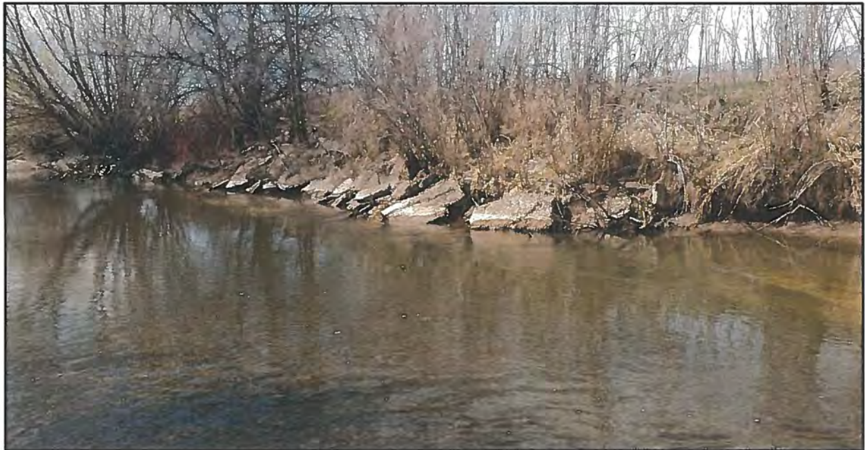
Photo 6: Concrete rubble used to armor banks, cobbles, and gravel common to native stream bed
