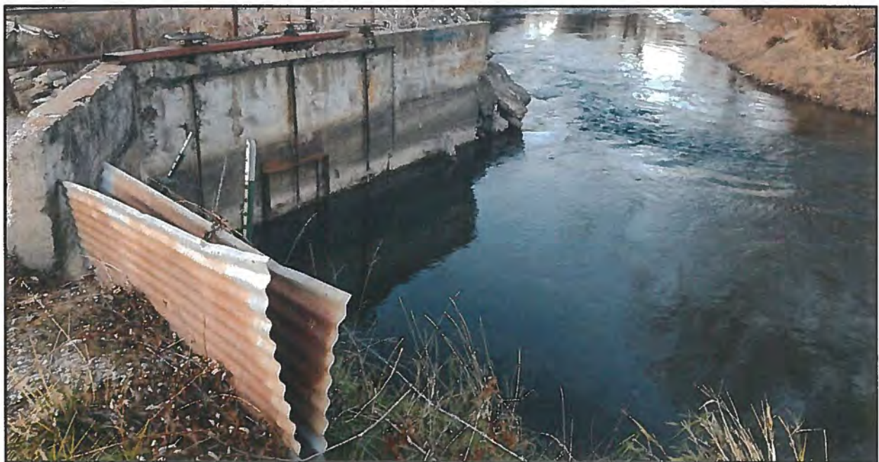
Photo 2: Existing diversion structure showing the river to the right without a check and sheet metal to prevent overtopping
