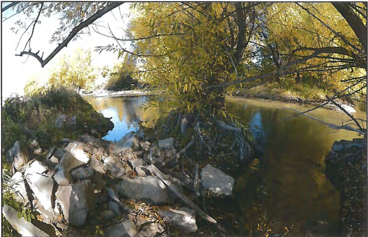
Photo 4: Crack willows growing into the channel with concrete piled around it to stop erosion
