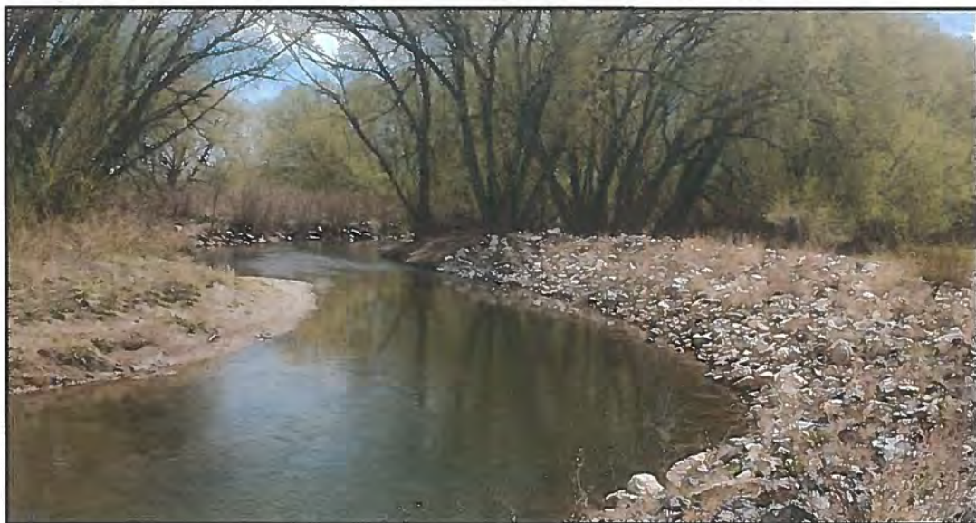
Photo 11: Unvegetated riprap bank scar that provides little-to-no habitat
