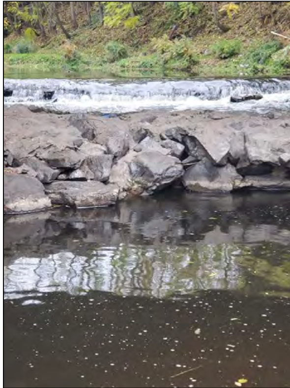
Photo 3 (September, 2021): Structure #2 (rubble) standing downstream looking upstream.
