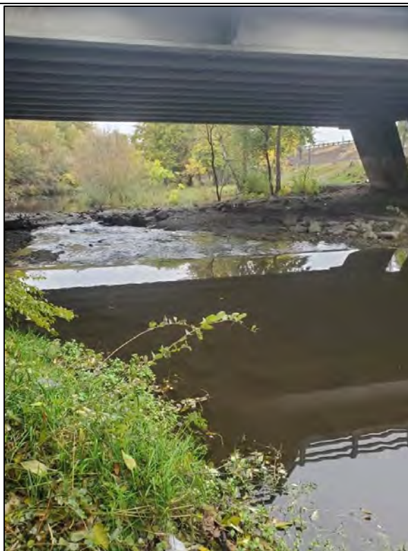
Photo 4 (September, 2021): Structure #2 (sewer line) in foreground and structure #2 (rubble) in background standing upstream looking downstream.
