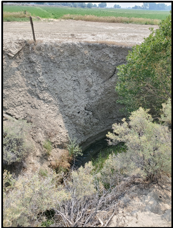
Photo 2 Erosion Caused by Tailwater from the D52 Lateral
