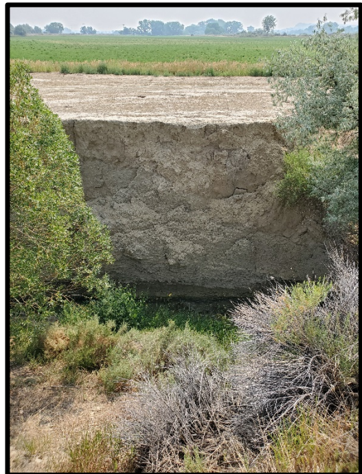
Photo 3 Significant Erosion Caused by Tailwater from the D52 Lateral
