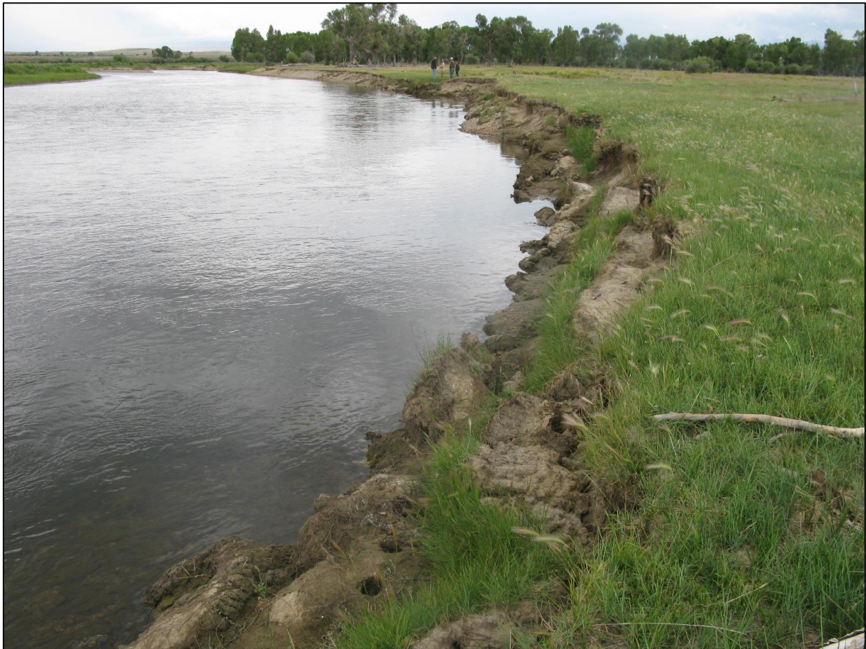
Photo 1: Eroding and sloughing stream banks like this one are common throughout the New Fork Gas Wells site. Restoration actions will target these areas.
