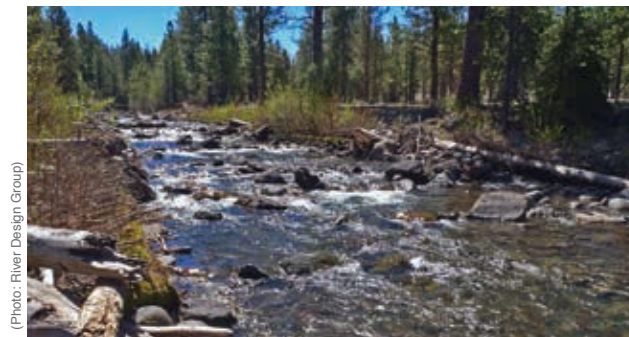
Wychus Creek, OR. A diversion structure that was a fish passage barrier (upper photo) was upgraded to provide fish passage by creating a "rock ramp" or engineered riffle (lower photo).
