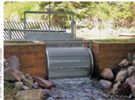
Morell Creek, OR. Both rotary drum (left) and flat panel screens were used on different diversions to prevent fish entrainment.
