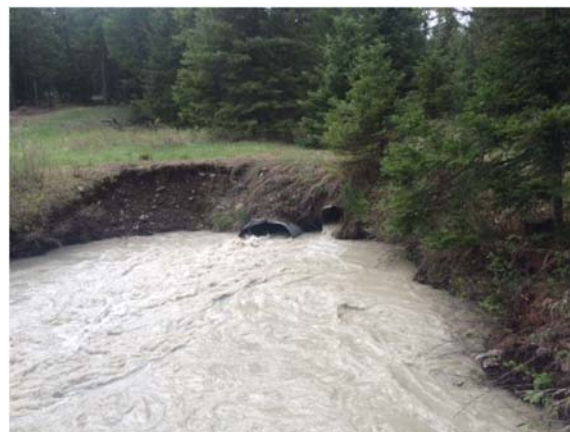
Figure 40. Undersized culvert during spring runoff.
