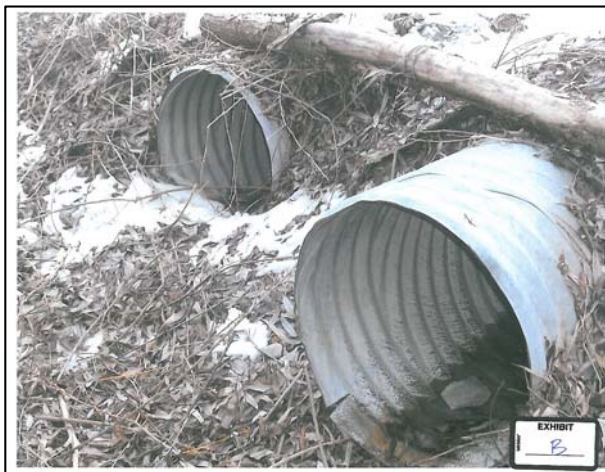
Figure 56. Undersized culverts at Olympia Way crossing before spring flow.
