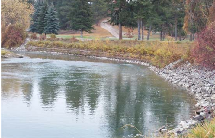
Figure 47. New willow lift along eroded shoreline on the Buffalo Hills property along the Stillwater River.
