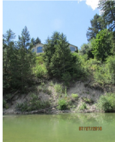
Figure 50. Mass failure of streambank on east shore of Stillwater River, across from the golf course under Juniper Bend housing developments.
