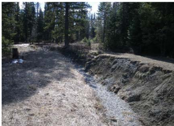
Figure 37. Krause Creek incising on lower reach before spring flow occurred, view from outside creek channel.
