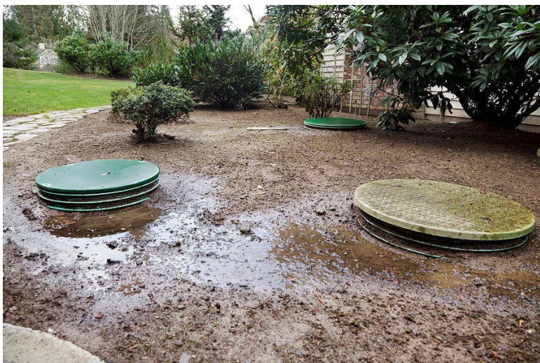
Figure 14. Leaking septic system in a residential yard. Surface leaks such as this can runoff over surfaces and impair nearby waterbodies ( www.hardwareandtools.com ).
