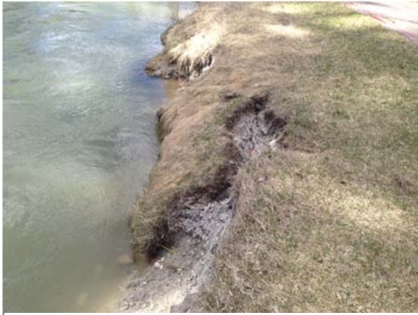
Figure 49. Bank undercutting and streambank erosion along cart path along the western shore of the Stillwater River.
