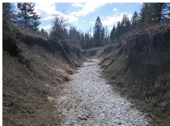
Figure 38. Krause Creek incising on lower reach before spring flow, view from inside the creek channel.
