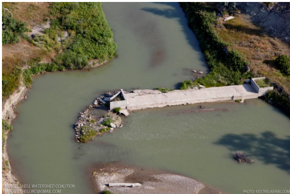
The Egge Diversion Dam was flanked by the 2011 flood.
