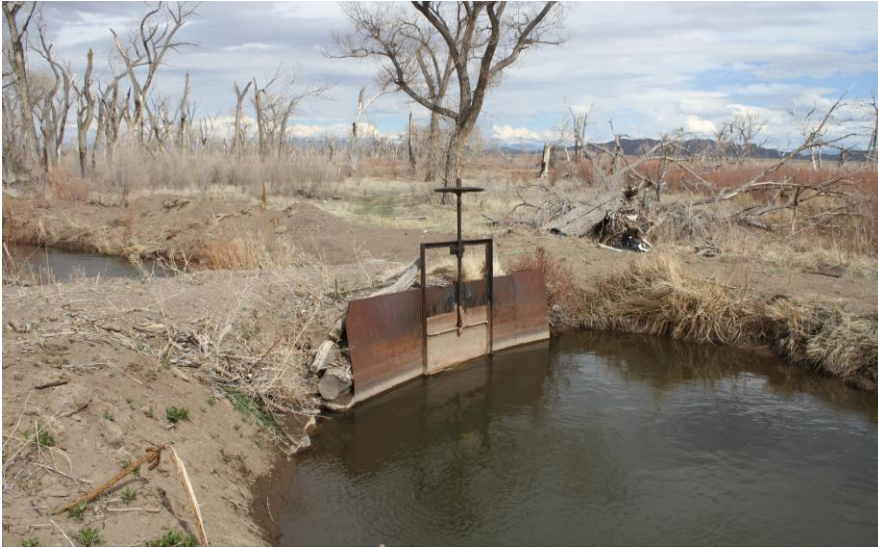
Figure 6: Poorly functioning William Stewart Co. Irrigation Ditch headgate.
