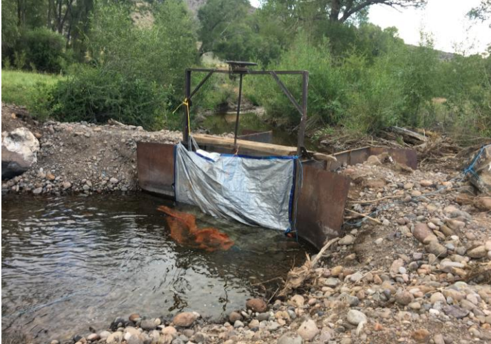
Figure 3: Erosion adjacent to the Mecitos Ditch headgate with temporary tarp installed to prevent leakage.
