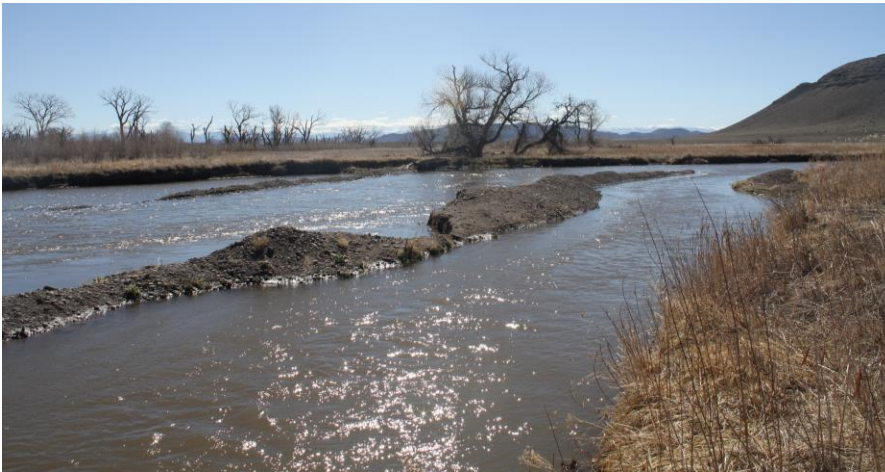
Figure 5: Poorly functioning diversion dam for the William Stewart Co. Irrigation Ditch.
