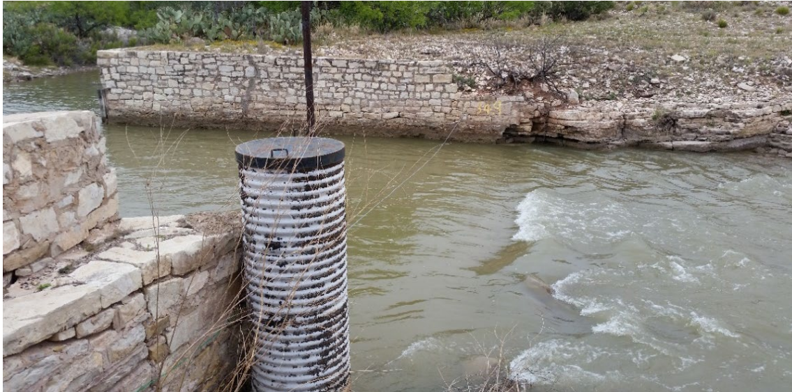
Figure 31. Aging infrastructure at CID (CID, all rights reserved).
