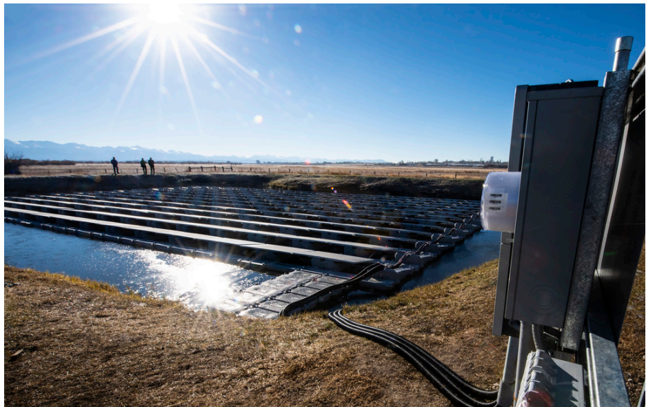
Figure 71. A photovoltaics installation by the State of Colorado in Walden, Colorado (Courtesy of the State of Colorado, all rights reserved).
