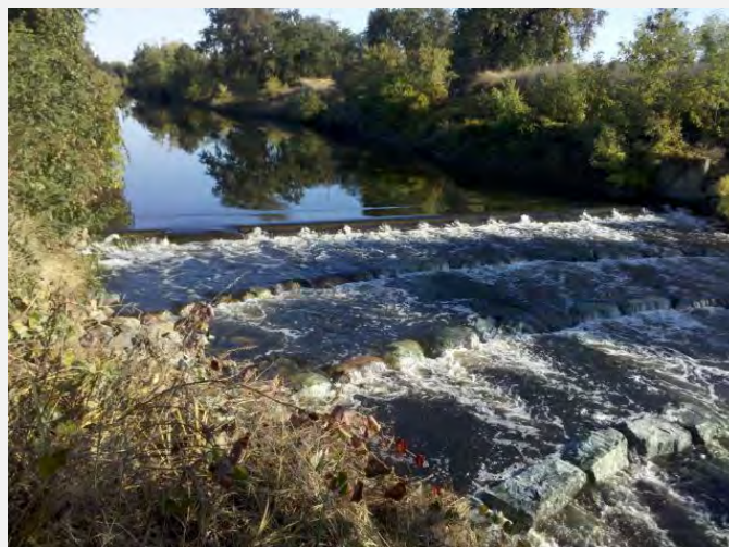
Figure 4: Flashboards installed on the Blodgett Dam.
