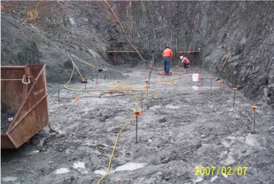
View of foundation following cleaning, acceptance and installation of screed stakes for the backfill concrete slab.
