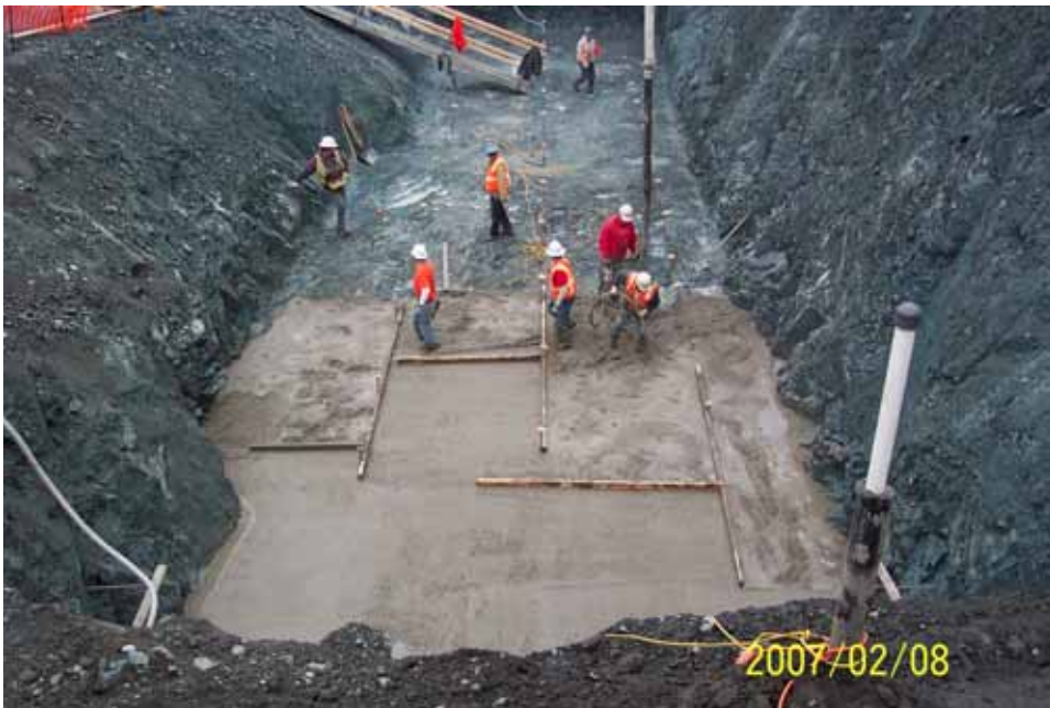
Placing backfill concrete leveling slab. The concrete is normal color and appears brown in contrast with the Greenstone.
