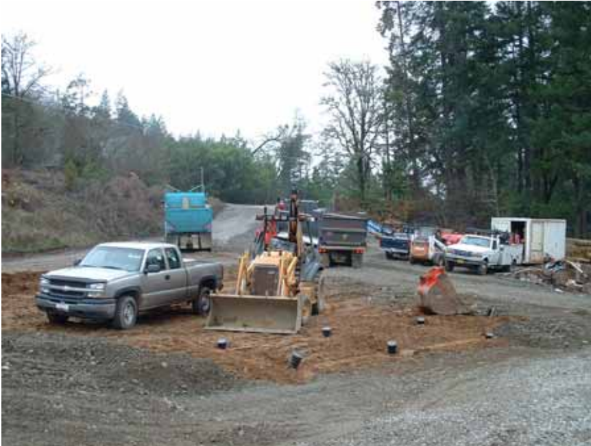
View of site access following installation of pipe arch and excavation for switch yard. 12/7/06
