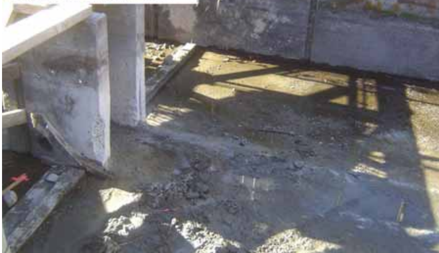
Savage Rapids Dam Removal and Replacement Pumping Plant - Contract 06SP101619 - View looking at downstream end of the Gravity Canal headworks following removal of pier. October 12, 2006 Photo by D. Stelma
