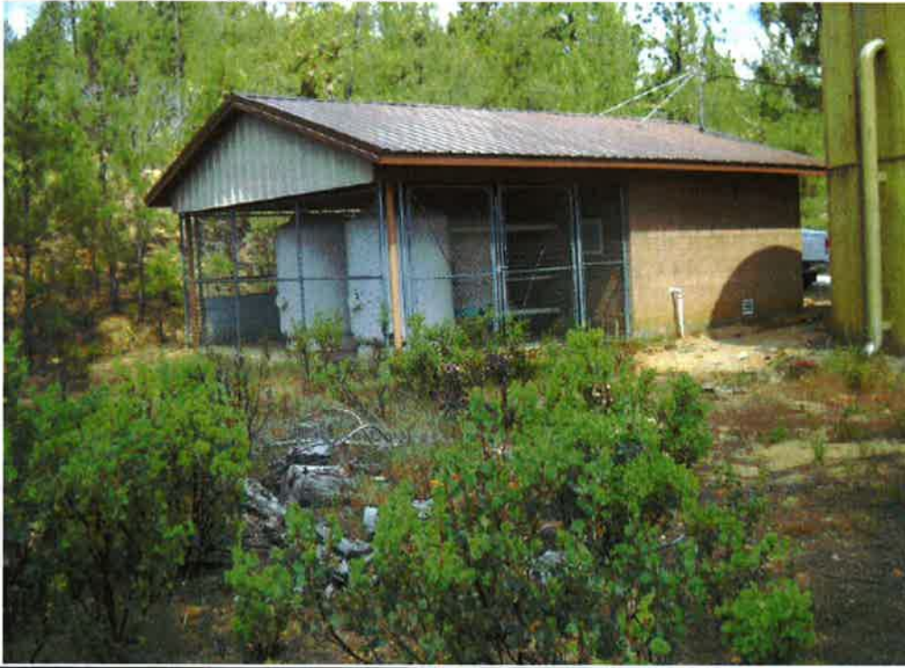
Existing wastewater treatment plant building. Roof overhang to be extended 8 feet to accommodate the additional filters (image from ENPLAN)
