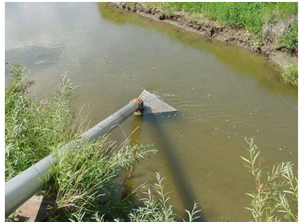
Submersible low water intake designed, constructed and demonstrated by NDSU for the Heart River Irrigators.
