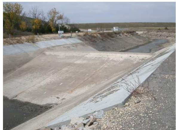
Broad crested weir constructed in spring of 2003 on Courtland Canal below Lovewell Dam in north-central Kansas
