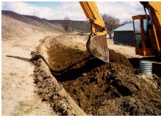
Belle Fourche ID, Angostura Unit, SD - Replacing open lateral with buried pipeline
