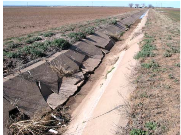
Typical damaged concrete lined section at Tom Green
