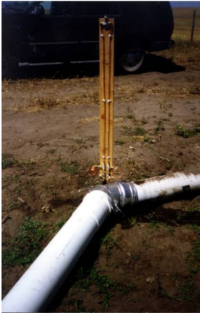
Field demonstration of inexpensive elbow meter at Mirage Flats Irrigation District
